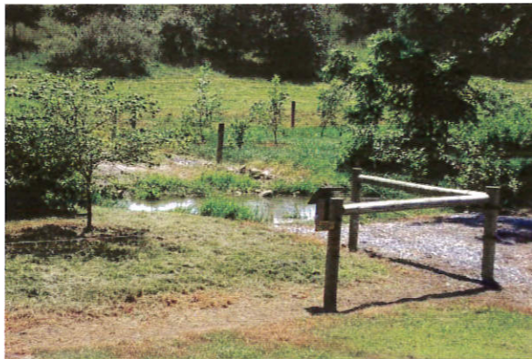
(Stream Bank Restoration with Cattle Crossing, Landes Farm, Marsh Run Project, Oct. '02)
