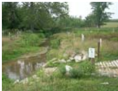
A freshly planted buffer installed at the Graver farm in Lancaster County.
